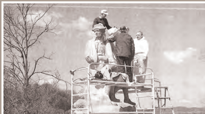
April 1962: Fred Mitchem (far right) supervising attachment of the center standing pioneer's replacement head he carved from matching sandstone.
