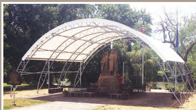
June 2020: Temporary cover installed by the City of Marietta using $50,000 Block Grant Funding.
